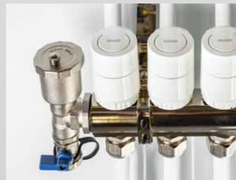
The room thermostat also controls valve drives (230 volt), which are mounted in the heating manifold.
