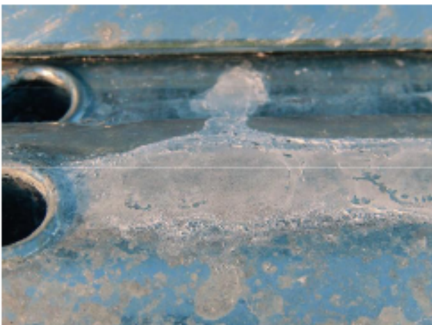
Image 3, White rust caused by water lying on the surface.
